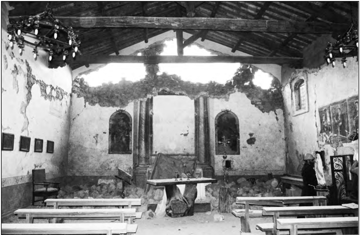
Figure 1 - Damages at the altar wall in the San Martino Church (Moletano, Amatrice) after the first shock of the 24th August 2016 [Photo credit: Diana L.]
